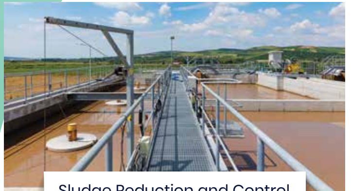
Sludge Reduction and Control
